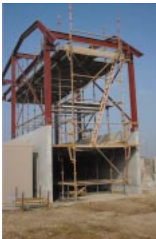
Woodchip store under construction. An automatic grab will carry woodchips to the gasifier hopper, part of the CHP plant
