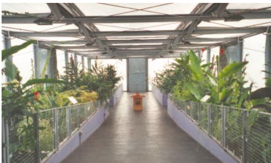
Waste water from domestic uses and sewage will be treated on-site with an intensive greenhouse-based reed system (photo of reed water treatment system at the Earth Centre, Doncaster)
