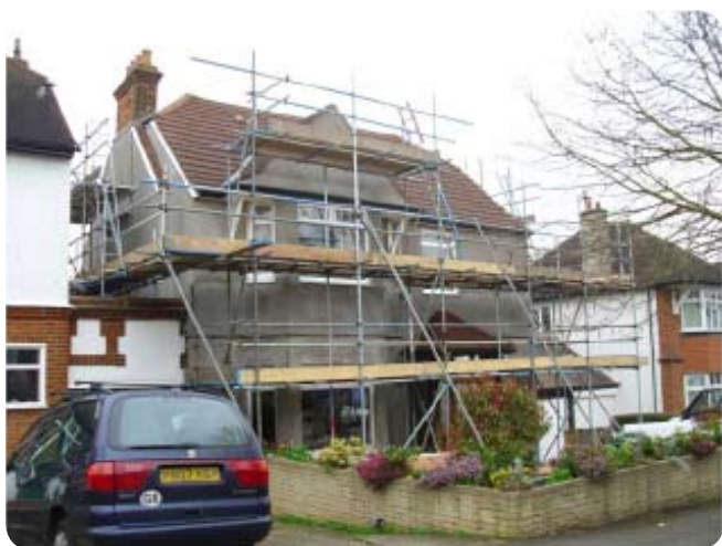
Step 2: Insulation and render is applied to the front and side of the property ready for finishing.
