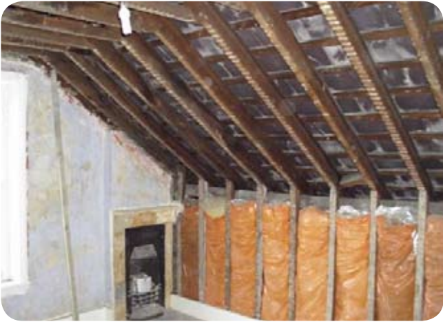
Before: Room in roof prior to insulation. Rafters are bare with minimal insulation.
